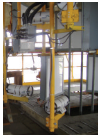
The automated, computer visioning system performs a 360 degree daily visual inspection of a rope with the hoist travelling at up to 20 metres a second.
